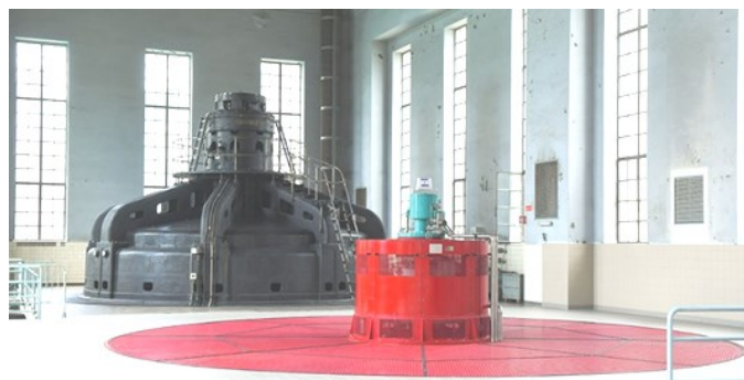
Turbine- rouge- Kaplan (2004 ) et turbine- noire-Francis (1925) photo SFMCP
